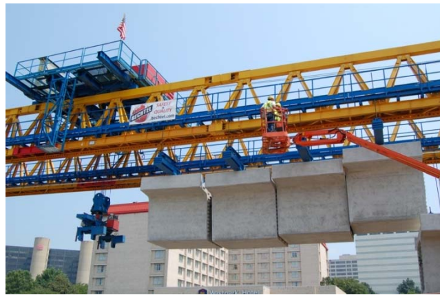
A horizontal crane is being used to build portions of the bridges for rail tracks in the middle of Route 7. Photo: Shea Daugherty, Dulles Transit Partners
