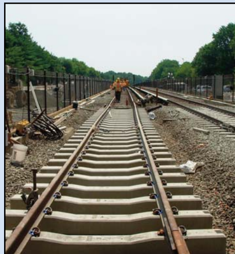
Crews are now laying track for the future Dulles Corridor Metrorail Project. Photo by Chuck Samuelson, Dulles Corridor Metrorail Project
