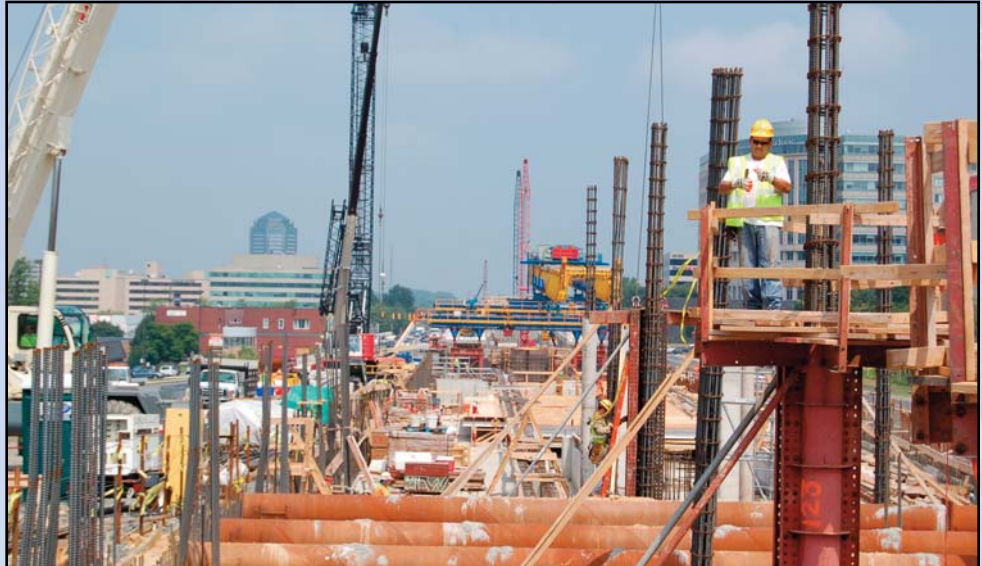
A view from inside the Tysons Central 7 Station, facing west. Crews are pouring foundation slabs and building columns. The truss building the Tysons West guideway is in the distance, just before the Westpark/Gosnell intersection. Photo by Shea Daugherty, Dulles Transit Partners
