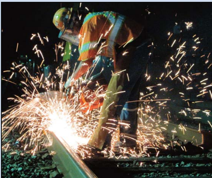
A welder performing critical work at the Orange Line tie-in during one of two July 2011 outages. Photo by John Green, Dulles Transit Partners
