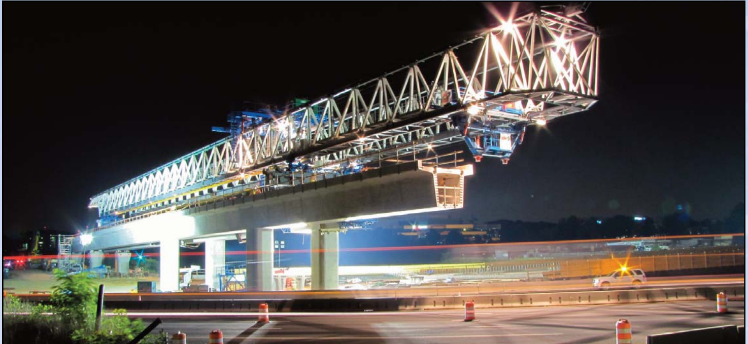
HIGH ABOVE I-495: A horizontal crane continues to be used to build bridges across the busy Capital Beltway in Tysons Corner. Photo by Chuck Samuelson, Dulles Corridor Metrorail Project
