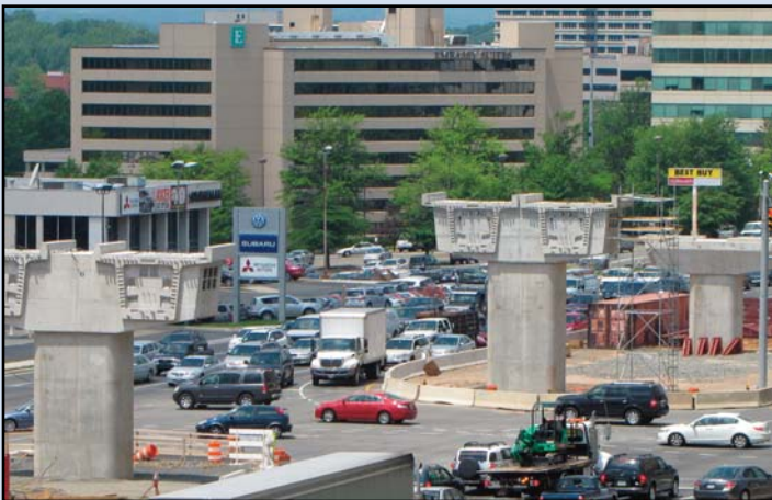
ALONG ROUTE 7: Pier construction takes place along Route 7 at the Gosnell/West-Park intersection. Photo by Chuck Samuelson, Dulles Corridor Metrorail Project
