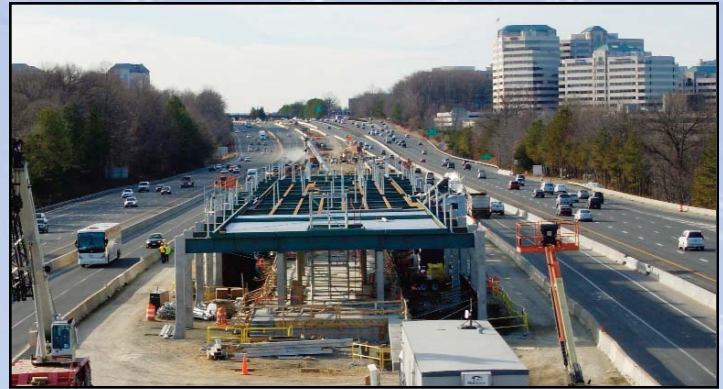
WIEHLE AVE: The Wiehle Avenue Metrorail Station is now 28 percent complete. Photo by Stephen Barna, Dulles Corridor Metrorail Project
