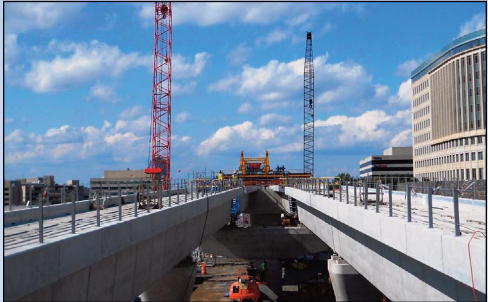
IN THE MEDIUM OF ROUTE 7: This photo shows the Sept. 29 view rising out of the Tysons Central 7 Metrorail Station looking west along the Tysons West Guideway. Photo by Stephen Barna, Dulles Corridor Metrorail Project
