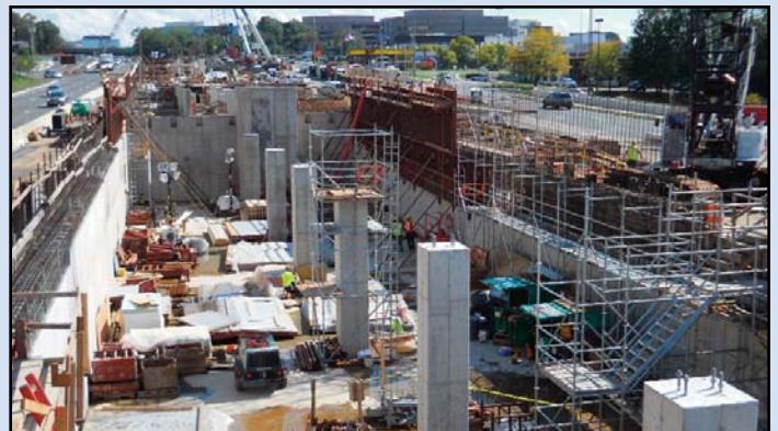
POWER FOR RAIL: Pictured is Traction Power Substation 5 at the Tysons Central 7 Metrorail Station. It is being built below the station platform deck. Retaining walls on both sides are in various stages of completion in preparation for structural steel framing. Photo by Stephen Barna, Dulles Corridor Metrorail Project
