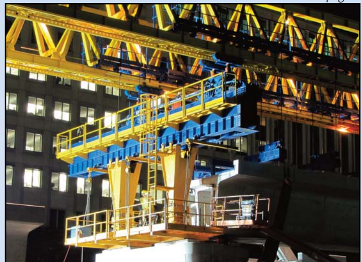
ABOVE ROUTE 7: Crews work to build bridges in the median of Route 7, using a large yellow and blue horizontal crane to lift concrete segments into place. Photo by Chuck Samuelson, Dulles Corridor Metrorail Project
