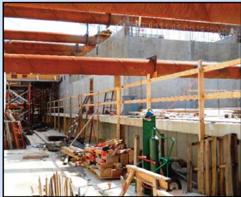
SUPPORT SYSTEMS: Platform walls and deck and the train control room and walls of an ancillary room are complete along a section of trackway. Photo also shows installation of towers for a fan room. Photo by Stephen Barna, Dulles Corridor Metrorail Project
