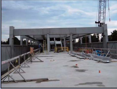
AT WIEHLE AVENUE: Looking east from the west end of the station platform, the concrete cladding of the steel framing for the mezzanine is complete. Photo by Stephen Barna, Dulles Corridor Metrorail Project
