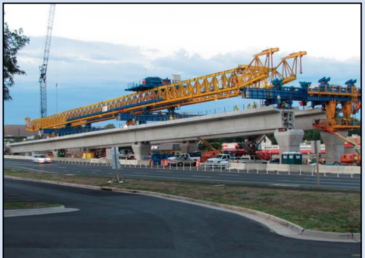
ALONG ROUTE 7: This horizontal crane is building bridges in the median of Route 7 working near the Gosnell/Westpark intersection. Photo by Chuck Samuelson, Dulles Corridor Metrorail Project
