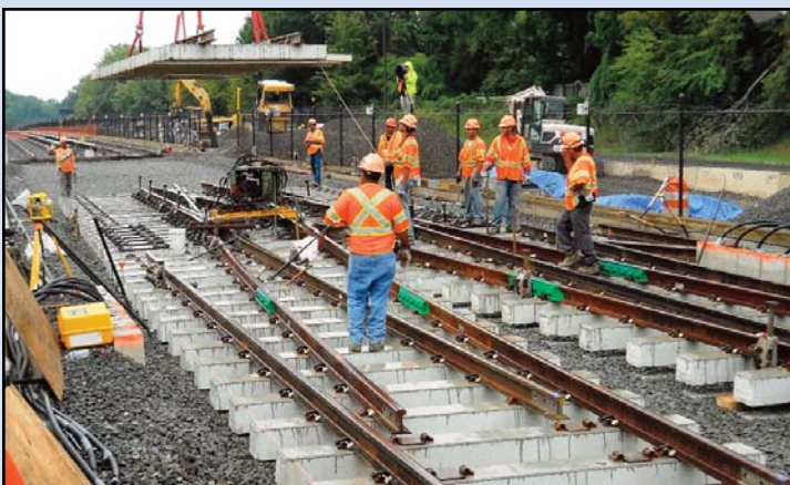
INTO PLACE: Crews lift and place a double crossover panel where existing tracks have been removed. Photo by Stephen Barna, Dulles Corridor Metrorail Project
