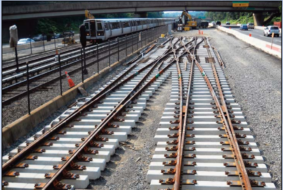
TYING IN THE ORANGE LINE: Double crossovers just before installation over Labor Day weekend looking west-bound in the median of Interstate 66. Photo by Stephen Barna, Dulles Corridor Metrorail Project
