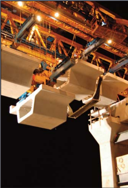
IN THE AIR: Crews are working to complete portions of the aerial guideway along Route 123 between the Dulles Connector Road and Interstate 495 near the Capital One complex. Photo by Shea Daugherty, Dulles Transit Partners
