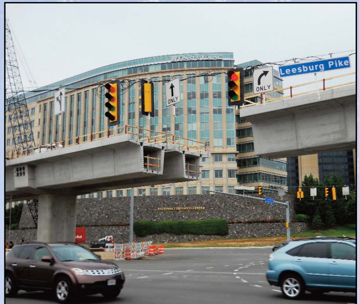
CROSSING GOSNELL/WESTPARK: The cantilevered segmental construction span at the intersection of Route 7 and Gosnell Road continues. Photo by Stephen Barna, Dulles Corridor Metrorail Project
