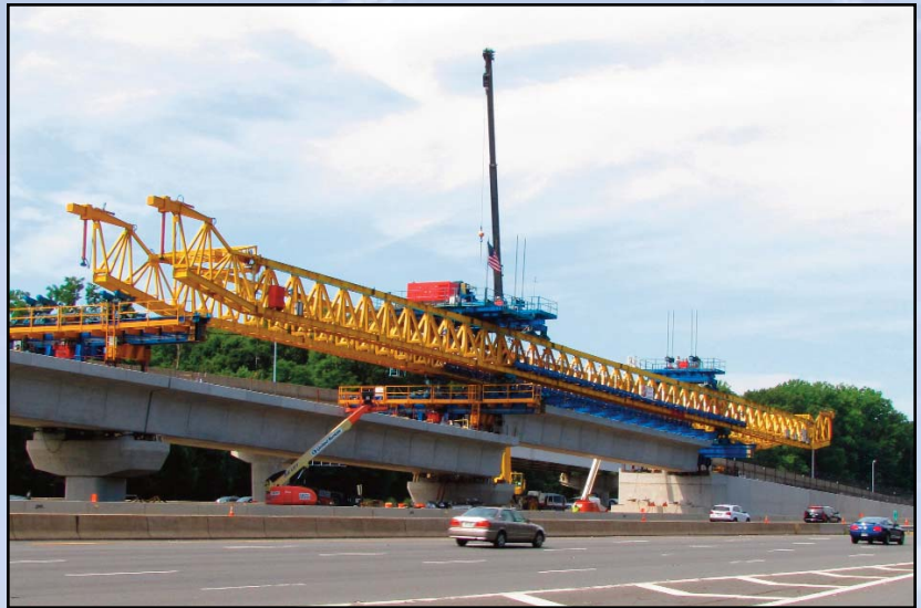
NEARING THE FINISH LINE: The final span in the bridges for rail in Tysons is poised for installation in the median of the Dulles International Airport Access Highway/Toll Road corridor just west of the Route 7 interchange. Photo by Chuck Samuelson, Dulles Corridor Metrorail Project
