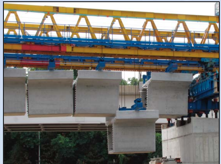
LIFTING SEGMENTS: Crane lifts segments for bridge spans along the Dulles Airport Access Highway/Dulles Toll Road near Route 7. Photo by Chuck Samuelson, Dulles Corridor Metrorail Project
