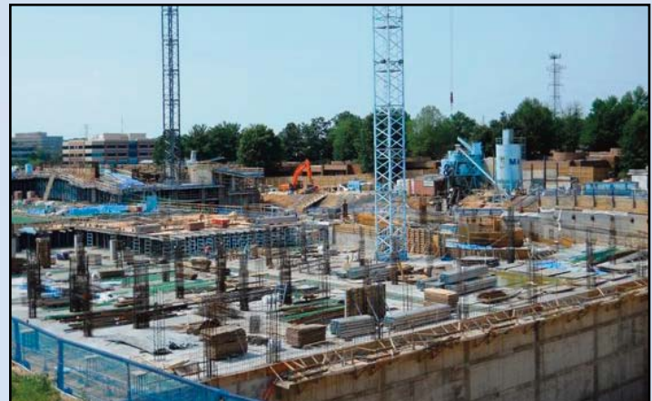
AT WIEHLE AVENUE: The Fairfax County/Comstock joint venture development has completed the excavation for the lower level parking decks that serve the Wiehle-Reston East Station. Photo by Stephen Barna, Dulles Corridor Metrorail Project
