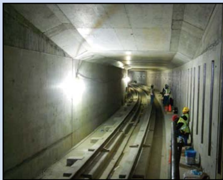
LET THERE BE LIGHT: Crews install light fixtures and conduit in the inbound and outbound tunnels that will be carrying trains from Route 123 to Route 7. Photo by Stephen Barna, Dulles Corridor Metrorail Project
