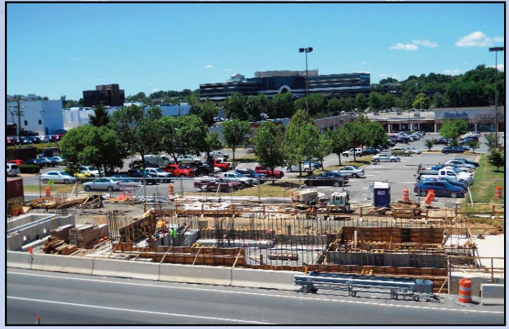
A SOUTHERN VIEW: This view of the construction of the concrete foundation and reinforcing steel installations for wall at the Greensboro Station (formerly the Tysons Central 7 Station) shows proximity of the station to the Marshalls/Home Goods/Sports Authority shopping center. Photo by Stephen Barna, Dulles Corridor Metrorail Project
