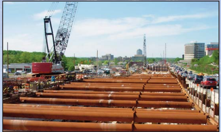
ON TOP OF THE TUNNEL: Cranes frame the view of the Sheraton Hotel in the distance in this photo looking west from the top of the cut-and-cover tunnel area along Route 7, leading to the future Tysons Central 7 Metrorail Station. Photo by Stephen Barna, Dulles Corridor Metrorail Project
