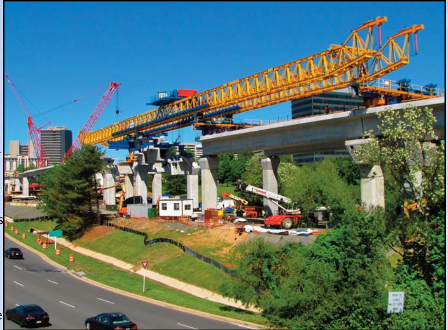
APPROACHING TYSONS CENTRAL 123: Construction continues on the bridges across Tysons Boulevard. Photo by Chuck Samuelson, Dulles Corridor Metrorail Project
