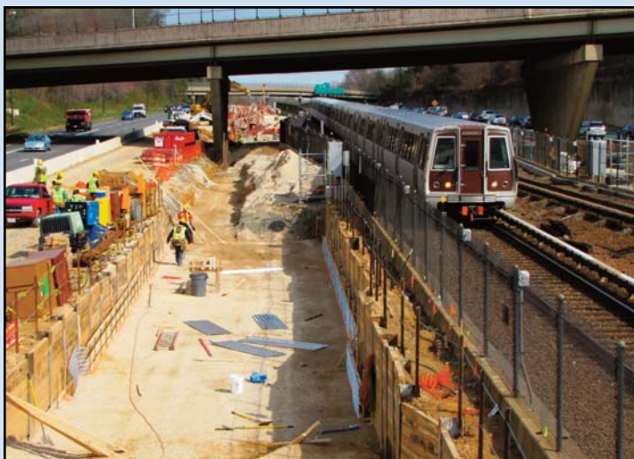
AT I-66: Construction continues close to Metro's Orange Line. Photo by Chuck Samuelson, Dulles Corridor Metrorail Project
