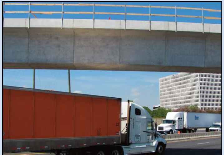
BRIDGES OVER THE BELTWAY: Lane closings on I-495, the Capital Beltway, are resuming as construction for the bridges for the future Dulles Corridor Metrorail line continues. Photo by Chuck Samuelson, Dulles Corridor Metrorail Project
