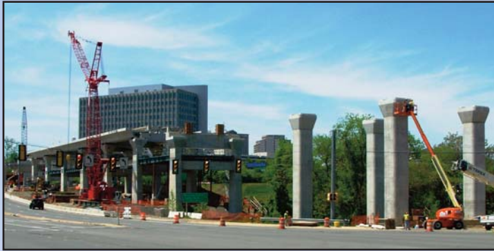
PROGRESS! PROGRESS!: Work continues on the Tysons East Station along Route 123 at Scotts Crossing. This will be the first stop on the westbound Dulles Rail extension. Photo by Stephen Barna, Dulles Corridor Metrorail Project
