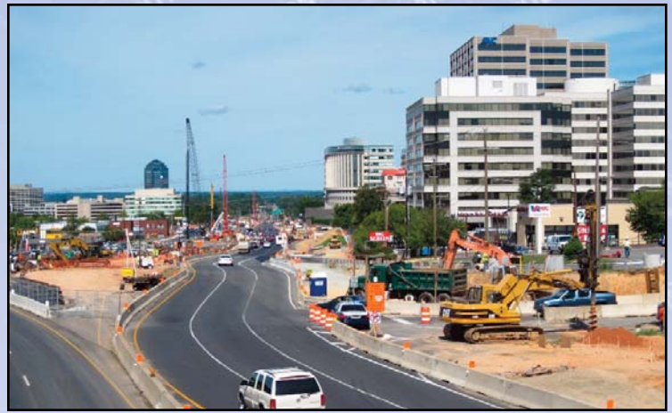
Construction of the Tysons Central 7 Station is progressing in the median of the eastbound and westbound lanes of Route 7 in Tysons Corner near the Route 123 interchange. Photo by Dulles Corridor Metrorail Project
