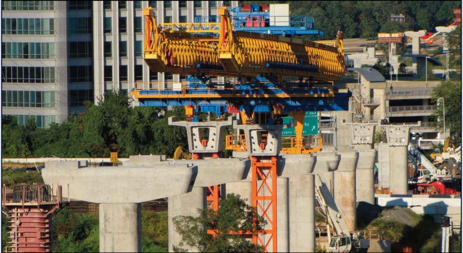
The giant blue and yellow truss now being used along Route 123 in Tysons Corner approaches I-495. Photo by Chuck Samuelson, Dulles Corridor Metrorail Project
