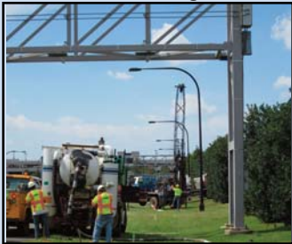
SAMPLES: Capital Rail Constructors crews perform geotech borings for pier locations along Saarinen Circle at Dulles Airport. Photo by Scott Evans, Dulles Corridor Metrorail Project
