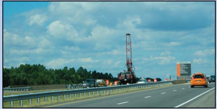
ALONG THE DULLES ACCESS HIGHWAY: Crews prepare for bridge abutments near Centreville Road. Photo by Scott Evans, Dulles Corridor Metrorail Project
