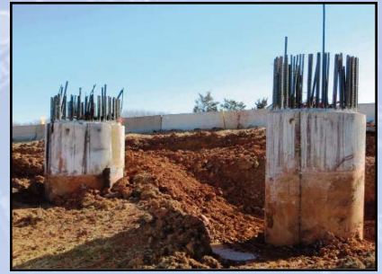
PHASE 2 CAISSON TEST SHAFT LOCATION #3: Excavating and exposing the test caissons four feet below grade in preparation for partial demolition. Photo by Steven Suddarth
