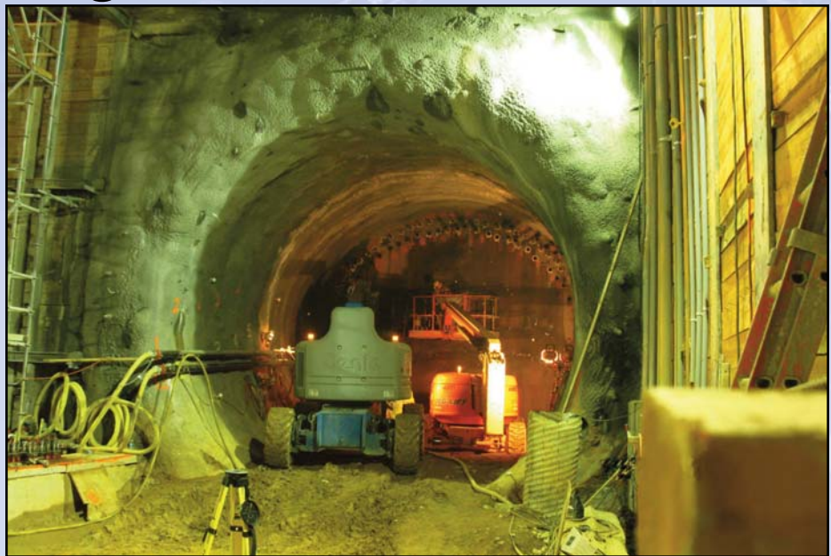
Construction of the 2,400-foot tunnel begins. The tunnel will connect Route 123 to Route 7 in Tysons Corner. Photo by Andrew Stone, Dulles Corridor Metrorail Project
