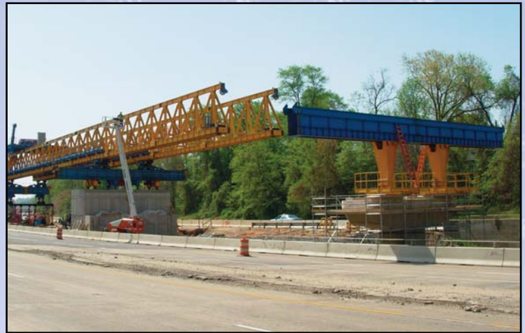
The first guideway span erection, taking place on the Dulles Connector Road at the Chain Bridge Road overpass. Photo by Stephen Barna, Dulles Corridor Metrorail Project
