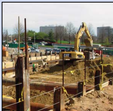
The Tysons Central 123 Metrorail Station construction is beginning, at the Route 123 and Tysons Boulevard intersection. Photo by Dulles Corridor Metrorail Project
