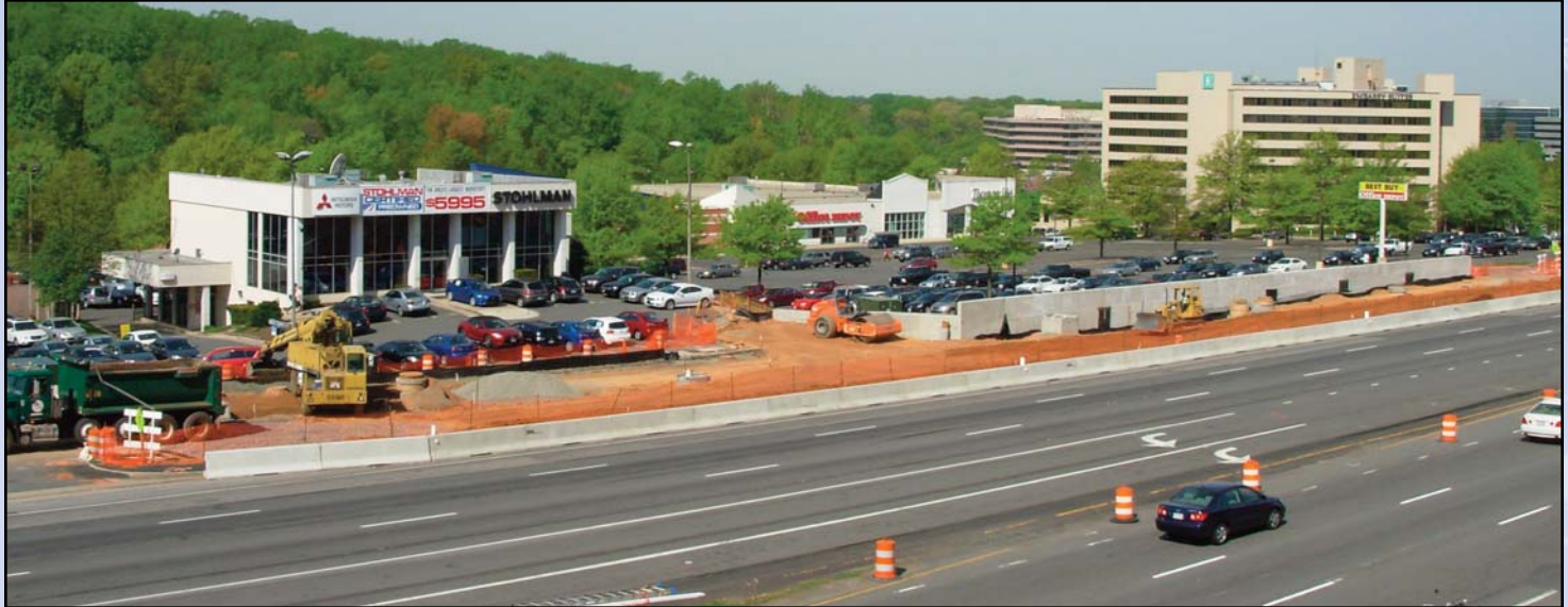
Retaining walls on Route 7, necessary to build up the service roads to the same grade as Route 7 for lane shifting. Photo by Stephen Barna, Dulles Corridor Metrorail Project
