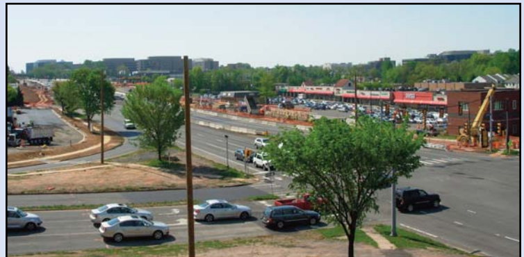
Route 7 retaining wall construction under way near the future Tysons Central 7 Metro Station. Photo by Stephen Barna, Dulles Corridor Metrorail Project
