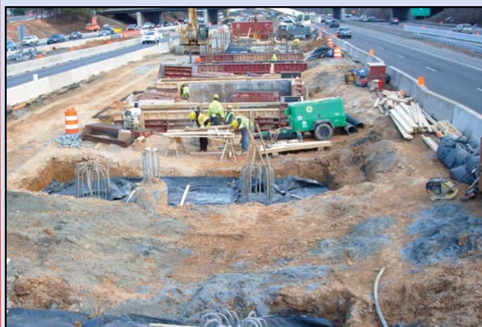
Caissons under construction for the foundations of the Wiehle Avenue Metro Station site. Photo by Dulles Corridor Metrorail Project
