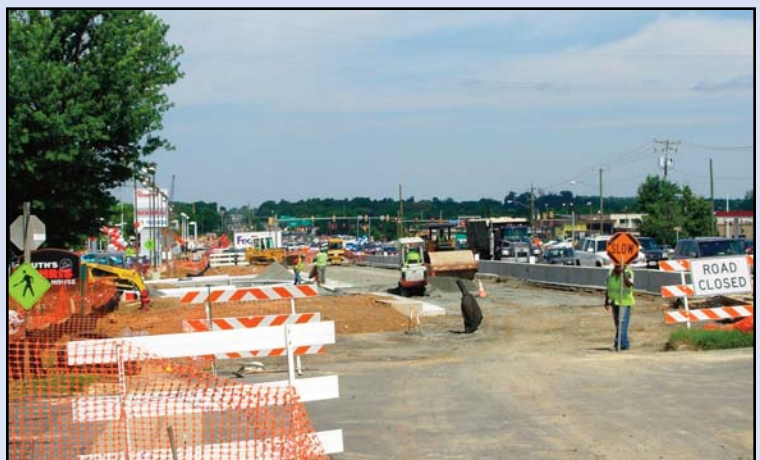
Crews work on the new eastbound lanes of Route 7 near the Nissan and Infiniti dealerships and Ruth's Chris Steak House where the roadway will be widened to make room for construction of the rail line and the Tysons West Metrorail Station just west of this area. Photo by Stephen Barna, Dulles Corridor Metrorail Project
