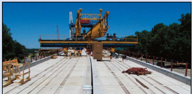
The first truss, located in the median of the Dulles Connector Road (Route 267) near the Route 123 intersection, continues guideway construction as it moves closer to Route 123. Photo by Dulles Corridor Metrorail Project
