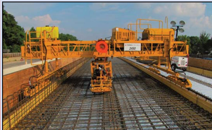
Civil crews have been working on several bridges over roads, trails and streams. This bridge work over Magarity Road in the median of the Dulles Connector Road (Route 267) is the beginning of some of the superstructure work, which requires massive amounts of rebar, concrete and system support. These bridges are part of the at-grade portions of the track that will eventually carry the future rail tracks. Photo by Chuck Samuelson, Dulles Corridor Metrorail Project
