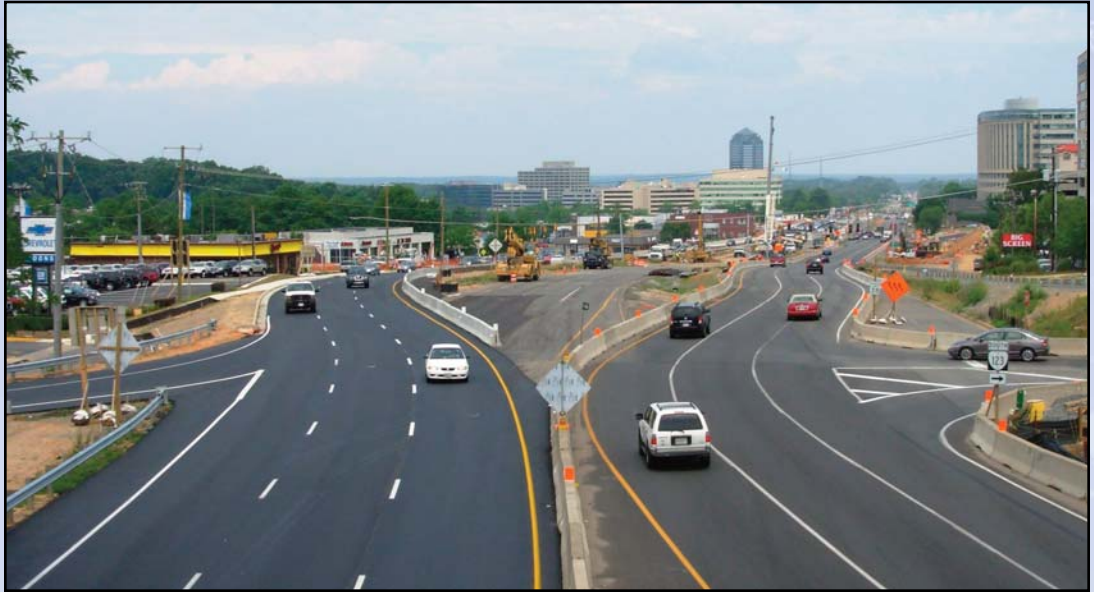
The newly shifted Route 7 to accommodate the Tysons Central 7 Station in the median, as seen from Route 123, in Tysons Corner. Photo by Stephen Barna, Dulles Corridor Metrorail Project
