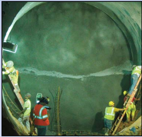
Miners working on the tunnels create dramatic underground scenes below the intersection of Routes 123 and 7. Photo by Dulles Corridor Metrorail Project
