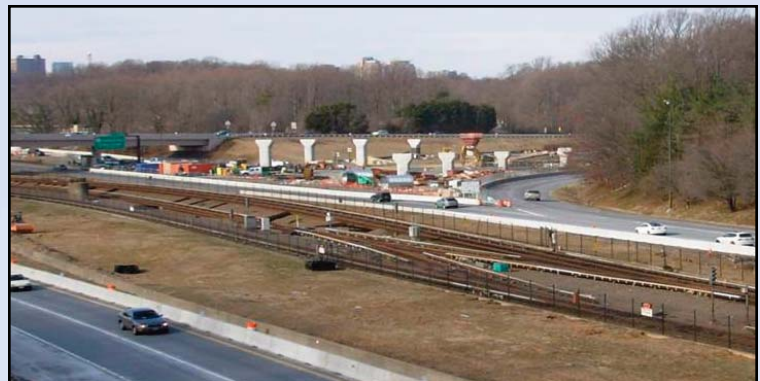
Pier guideway construction underway at the I-66 and Dulles Connector Road (Route 267) interchange. Photo by Dulles Corridor Metrorail Project
