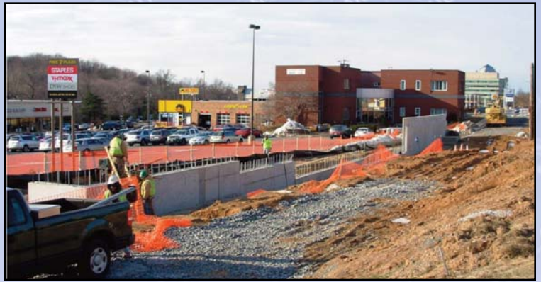
Construction of retaining walls on Route 7, necessary to build up the service roads to the same grade as Route 7 for lane shifting. Photo by Dulles Corridor Metrorail Project
