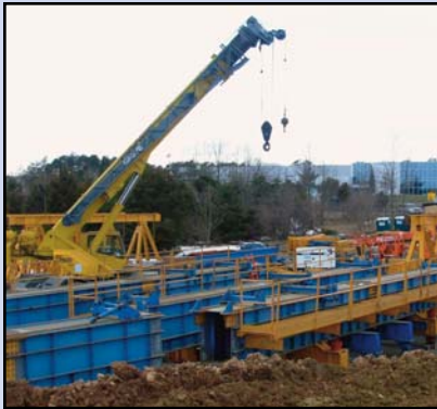
Truss assembly taking place at Dulles Airport. Soon, trusses will be all along the corridor as the guideways go up to support construction. Photo by Dulles Corridor Metrorail Project
