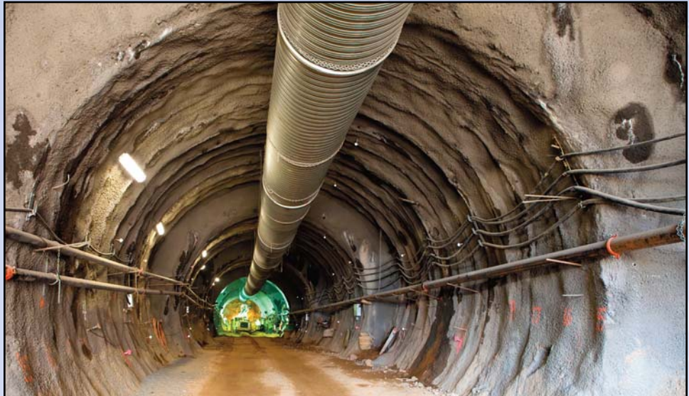
The outbound tunnel that will carry rail between Route 123 and Route 7 in Tysons Corner is currently 420-feet long and passes completely under International Drive. Photo by Rich Silva, Dulles Corridor Metrorail Project
