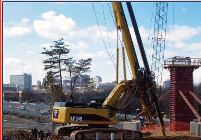
Pier construction at the Dulles Connector Road and Route 123 interchange leading up to the future Tysons East Station. Photo by Dulles Corridor Metrorail Project
