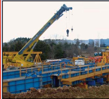
Truss assembly taking place at Dulles Airport. Soon, trusses will be all along the corridor as the guideways go up to support construction. Photo by Dulles Corridor Metrorail Project
