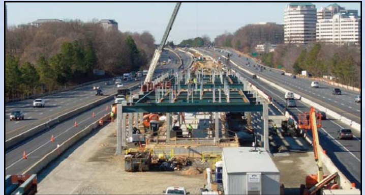
STATION CONSTRUCTION: Crews continue to work on the structural steel for the mezzanine. Photo by Chuck Samuelson, Dulles Corridor Metrorail Project
