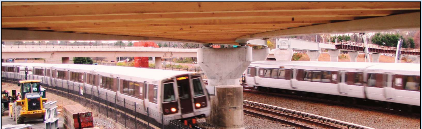
WORKING SIDE BY SIDE WITH METRO: Dulles Corridor Metrorail crews continue to work on the bridge spans for tracks above the existing Orange Line tracks near I-66 and the Dulles Connector Road (Route 267) where the rail extension will connect with the Orange Line. Photo by Chuck Samuelson, Dulles Corridor Metrorail Project
