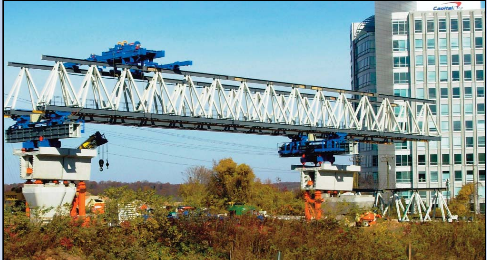
OVER THE BELTWAY: Construction begins to bring the Dulles Metro tracks over the Beltway in Tysons Corner using a white truss. Photo by Chuck Samuelson, Dulles Corridor Metrorail Project
