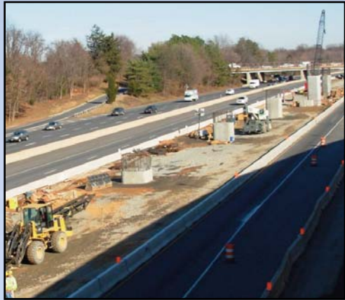
BRIDGE FROM ROUTE 7 TO TOLL ROAD MEDIAN BEGINS: Cranes are now driving piles to support the Tysons West guideway which will carry future trains from Route 7 to the median of the Dulles International Airport Access Highway and the Dulles Toll Road. To the right of this photo is the Sheraton Hotel and the Westwood Village residential community. On the other side of the highway behind the trees is the Carrington community. Photo by Dulles Corridor Metrorail Project
