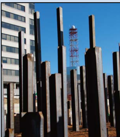
PREPARING FOR TYSONS CENTRAL 7: Piles to support the Tysons Central 7 Metrorail Station near SAIC in the foreground of the landmark communications tower at Route 7 and Route 123. Photo by Chuck Samuelson, Dulles Corridor Metrorail Project
