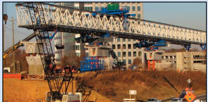
AIMING FOR THE BELTWAY: Crews are assembling the horizontal crane, also known as a truss, that will be used to build bridges for aerial tracks across the Capital Beltway starting in the Spring. Two other similar cranes are being used to build bridge spans from the Dulles Connector Road to Route 123 and have become familiar sights as the giant yellow and blue devices dominate the skies of Tysons. The new crane is white. Photo by Chuck Samuelson, Dulles Corridor Metrorail Project
