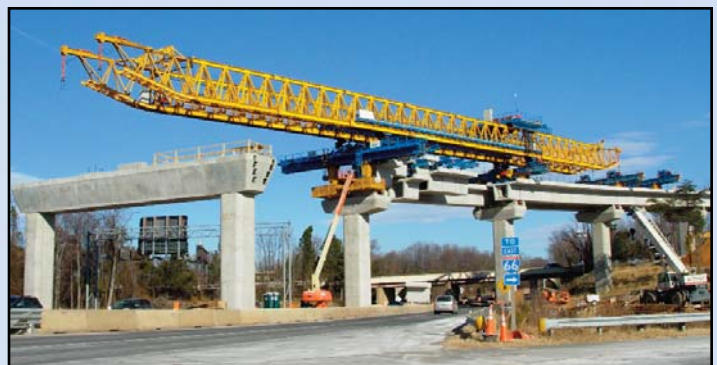
CROSSING ROUTE 123: The bridge construction at the Dulles Connector Road/Route 123 interchange is in the midst of reaching a major milestone, as the large truss has launched and is currently working over Route 123. This is another significant crossing for the truss, which has been commissioned since last Spring. Overnight closures of Route 123 should be expected when the bridge work is being performed overhead. Once this crossing is complete, the truss will continue moving westward, pier-to-pier, assembling bridge spans toward Scotts Crossing Road and the future Tysons East Metro Station. Photo by Chuck Samuelson, Dulles Corridor Metrorail Project
