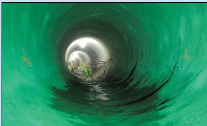
WATERPROOFING: Dulles Transit Partners crews continue with waterproofing operations inside one of the two tunnels that will carry tracks from the Tysons Central 123 Station at Route 123 and Tysons Boulevard to the Tysons Central 7 Station in the median of Route 7 just west of Route 123 near SAIC. Mining for both inbound and outbound tunnels was completed last year. Photo by Dulles Corridor Metrorail Project
