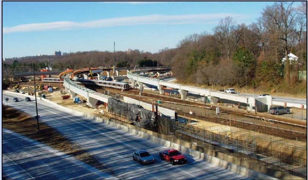
AT THE CONNECTING POINT: Girders have been set and more than 50 percent of the trackway concrete decks have been completed where the Dulles Corridor Metrorail Project's 23-mile extension of Metro's existing system joins the Orange Line tracks at I-66 and the Dulles Connector Road (Route 267). Photo by Chuck Samuelson, Dulles Corridor Metrorail Project
