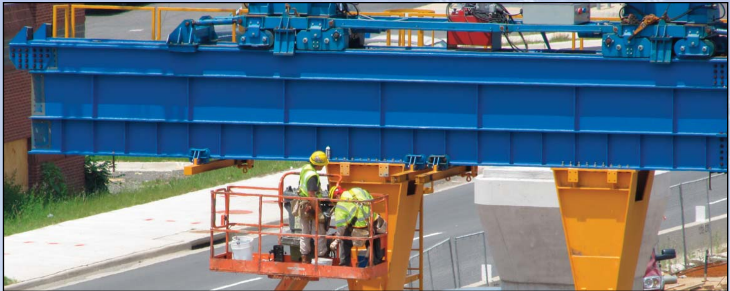
BUILDING BRIDGES ALONG ROUTE 7: Crews are now assembling a huge yellow and blue horizontal truss along Route 7 near the future Tysons Central 7 Metrorail Station. It is being used to build bridges for tracks west of this station. Photo by Chuck Samuelson, Dulles Corridor Metrorail Project
