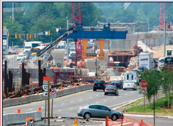
PIERS, PIERS, PIERS: Piers for the aerial guideway magnify the path for rail in the middle of Route 7. Photo by Chuck Samuelson, Dulles Corridor Metrorail Project
