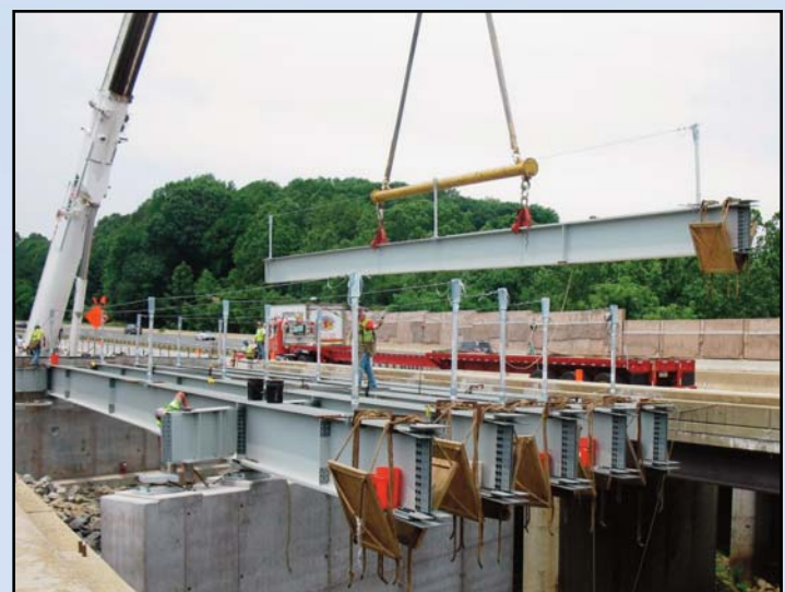
BUILDING THE DIFFICULT RUN BRIDGE: Crews erect steel girders between Pier 2 and Abutment 1 at the Difficult Run Bridge in the median of the Airport Access Highway/Dulles Toll Road. Photo by Geoff Griffith, Dulles Corridor Metrorail Project
