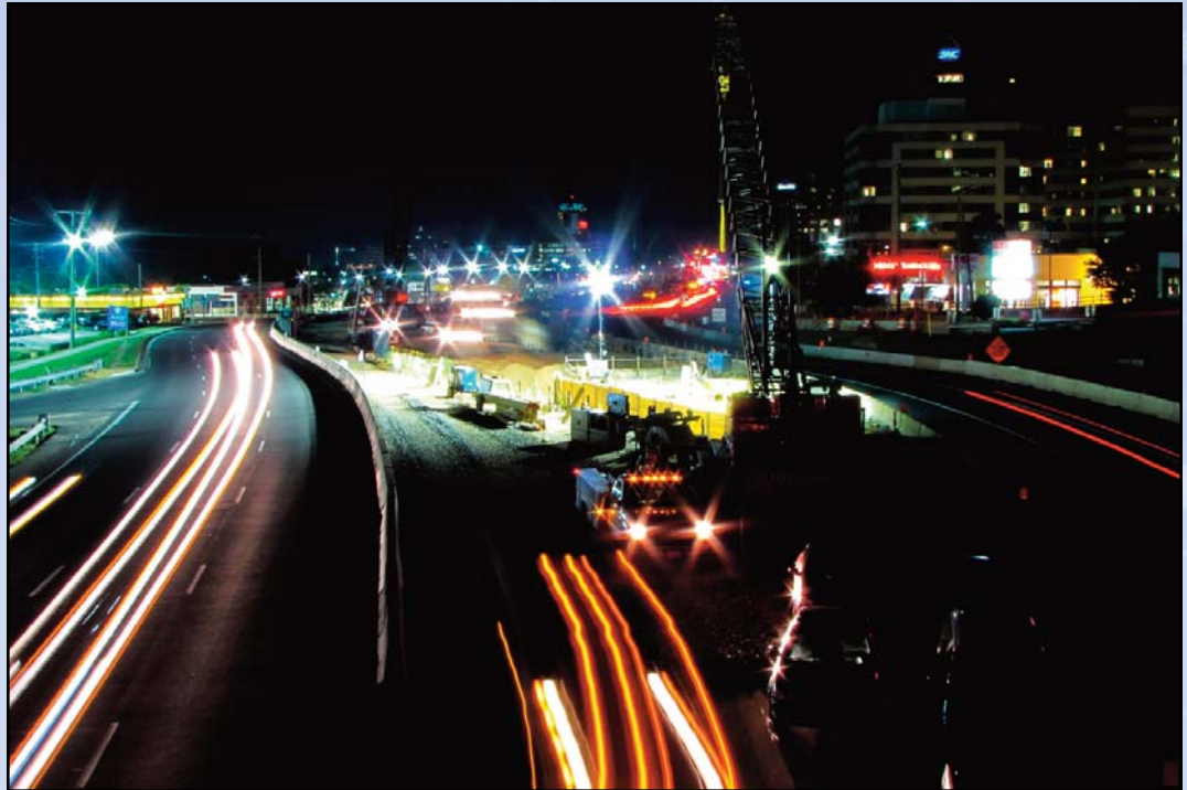
WORK HARDLY EVER STOPS: Construction changes Route 7 in Tysons at night. Photo by Chuck Samuelson, Dulles Corridor Metrorail Project
